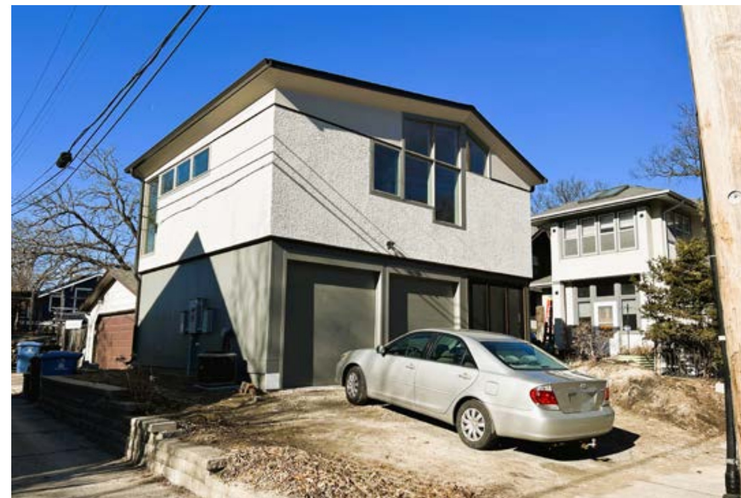
Windows are required on walls that face a public alley or street. This detached ADU has walls facing both a public alley and a street.
