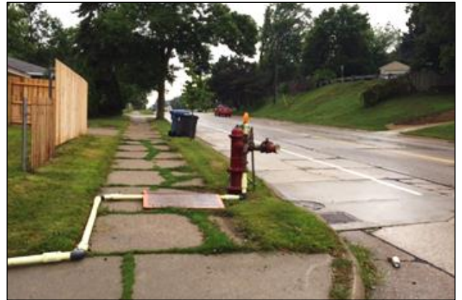
Temporary bypass piping set up in Minneapolis
