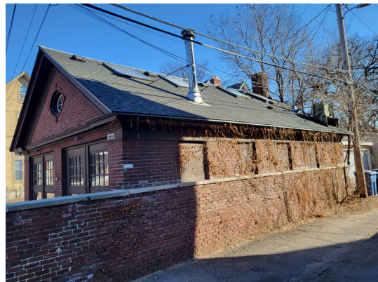
This carriage house at 2404 Stevens Ave has modern skylights and HVAC equipment on its rear roof slope. This location is not visible from the street.
