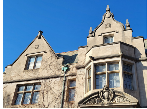
The house at 100 22nd St E has several historic roof features. The roof is covered with slate. The gutters are built into the roof. Stone parapets extend up from the roof. The one on the left is pointed. The one on the right is stepped and scalloped with carved finials.
