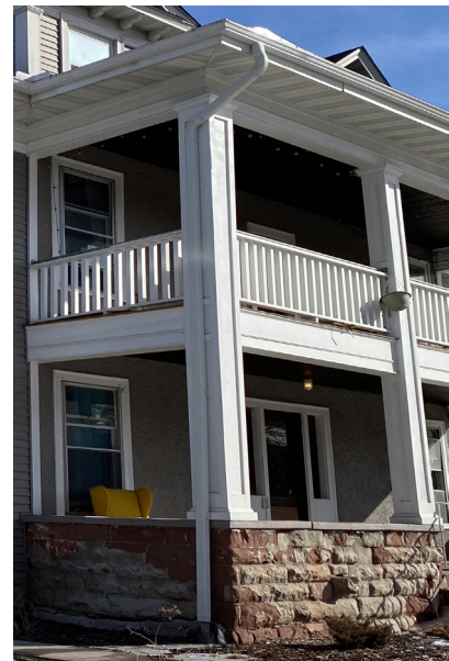
The square railing posts at 2511 1st Ave S are simple and do not mimic historic designs.
