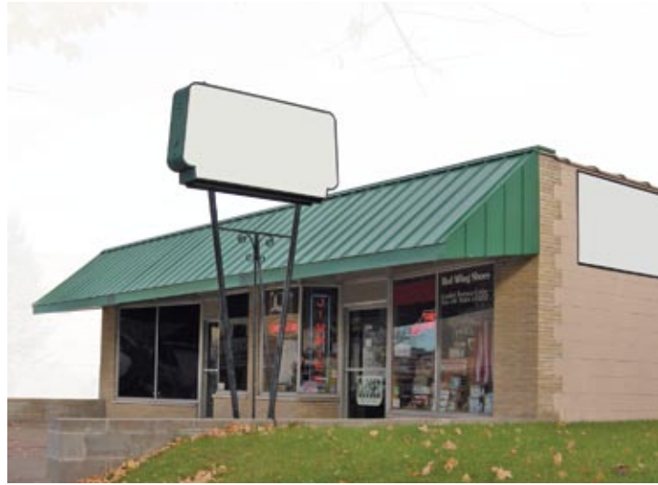
BEFORE This large metal awning overwhelms the small building.
