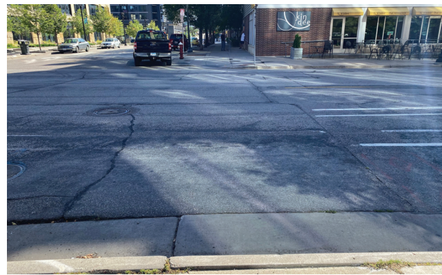
Poor pavement quality on 2nd Street
