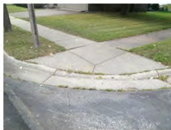
Some pedestrian ramps do not meet current ADA standards for accessibility.
