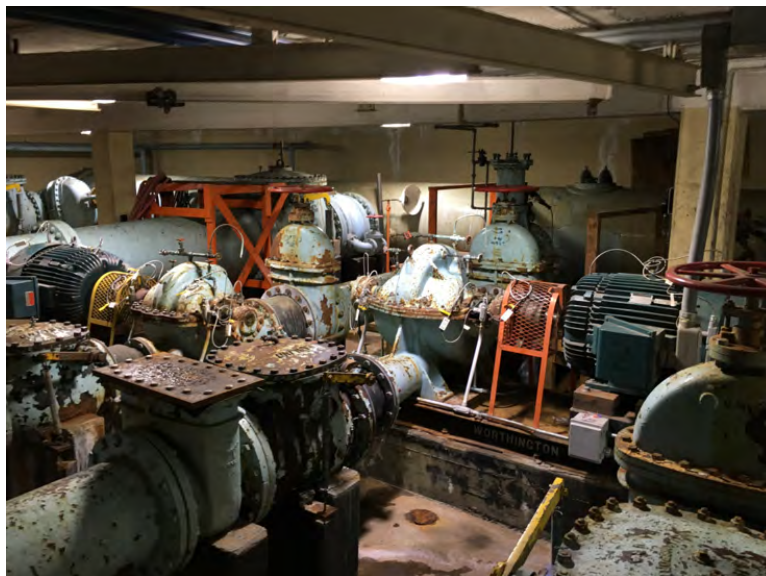
Picture of the Northeast High Service pumps.
